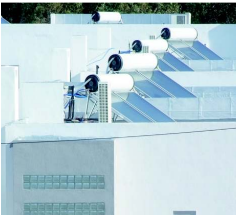
Installation solaire collective
